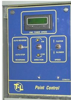
Point Control Panel
