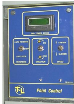
Point Control Panel
